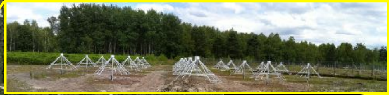
Mini-Array (MA) of 19 dual- polarization antennas
